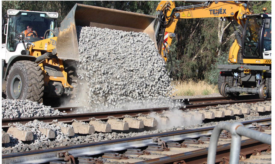
557,000 tonnes of locally sourced ballast has been used on the North East Rail Line Upgrade. New ballast has improved track stability and drainage, helping prevent new mud holes from forming.
