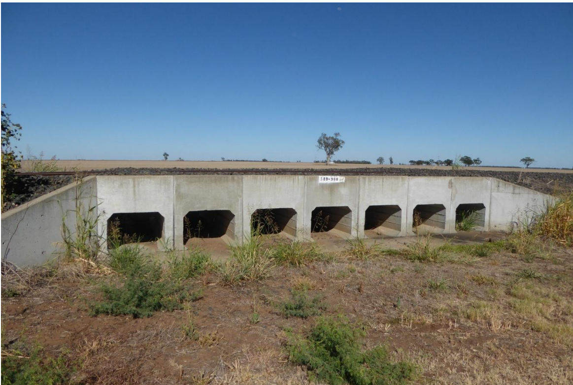
Figure 4.3 Photos of example culverts showing typical level of blockage – 589.3km
