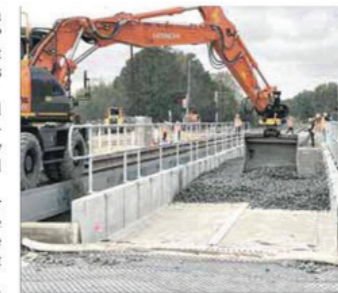
ON SCHEDULE: Works on the North East Rail Line are on track to be completed by 2021. Works include this rail bridge and level crossing construction and renewal undertaken in April of this year.
