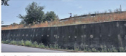
Spot Dave: The man dwarfed by the huge concrete retaining wall next to Benalla Station on Mackellar St is Benalla Rail committee member David Moore. Under ARTC plans for the inland rail project the new wall will reach above seven metres.
