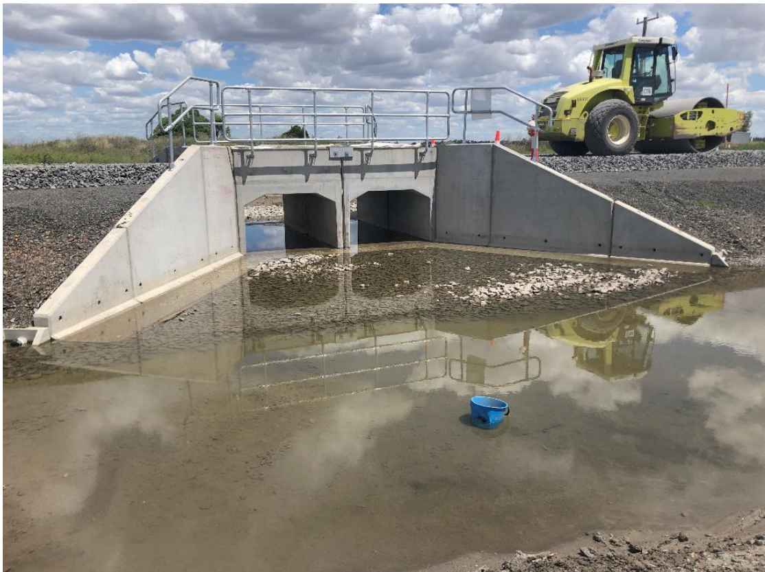
Plate 32 – Standing water under culvert in Roydon Road Crossing 686
