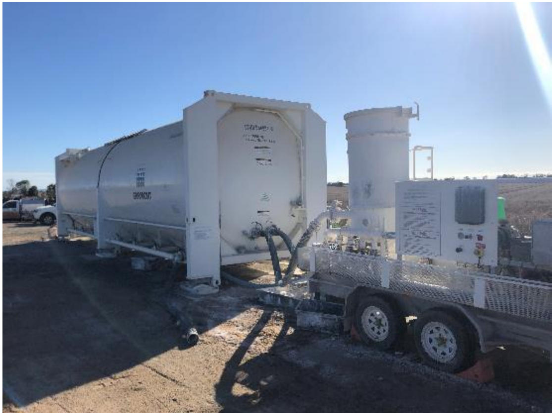
Plate 5 – Lime storage tank at Milguy MAF
