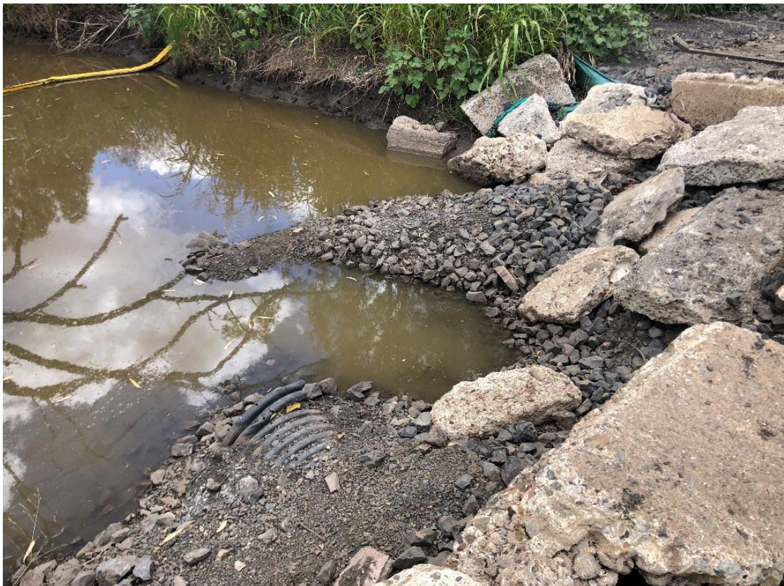
Plate 28 – Yallaroi Creek piling pad pipe blocked and evidence of scouring
