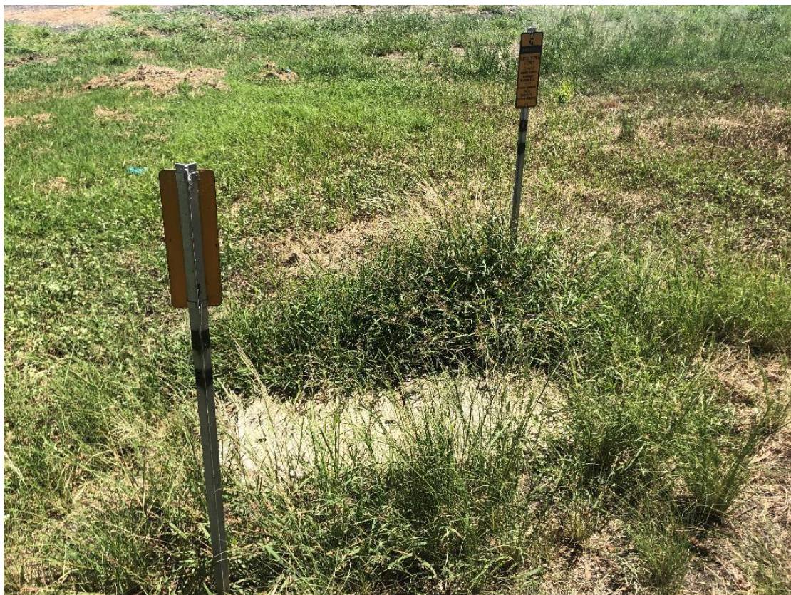
Plate 36 – Gurley Crossing Telstra pits
