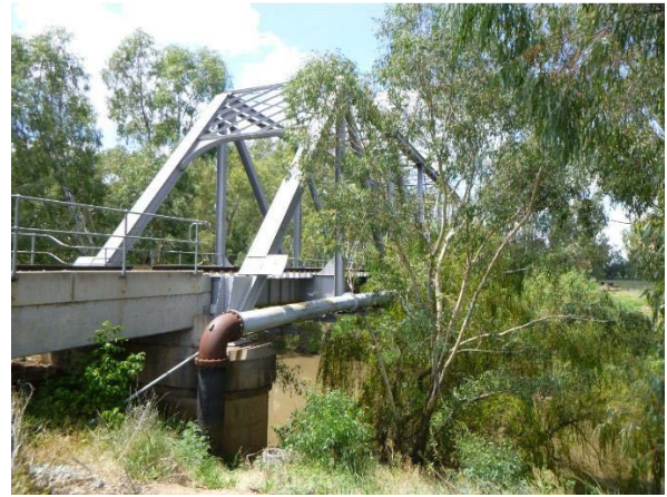
4. View of the water pipe along the western side of the bridge.
