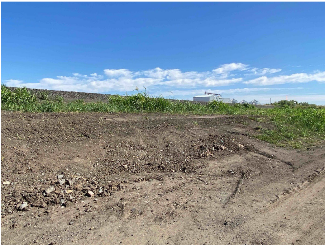
Plate 20 – Area along alignment not yet landscaped, with minor sediment runoff present, near Croppa Moree Road MAF
