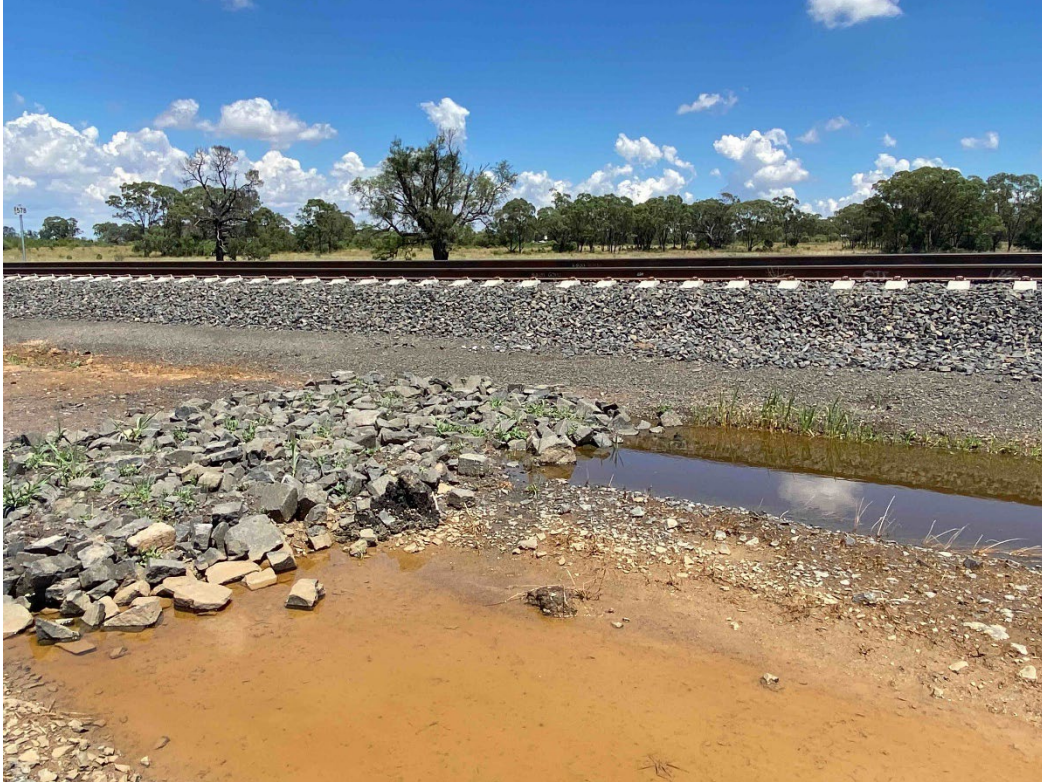
Plate 9 – Water pooling at scour protection at Gate 2.
