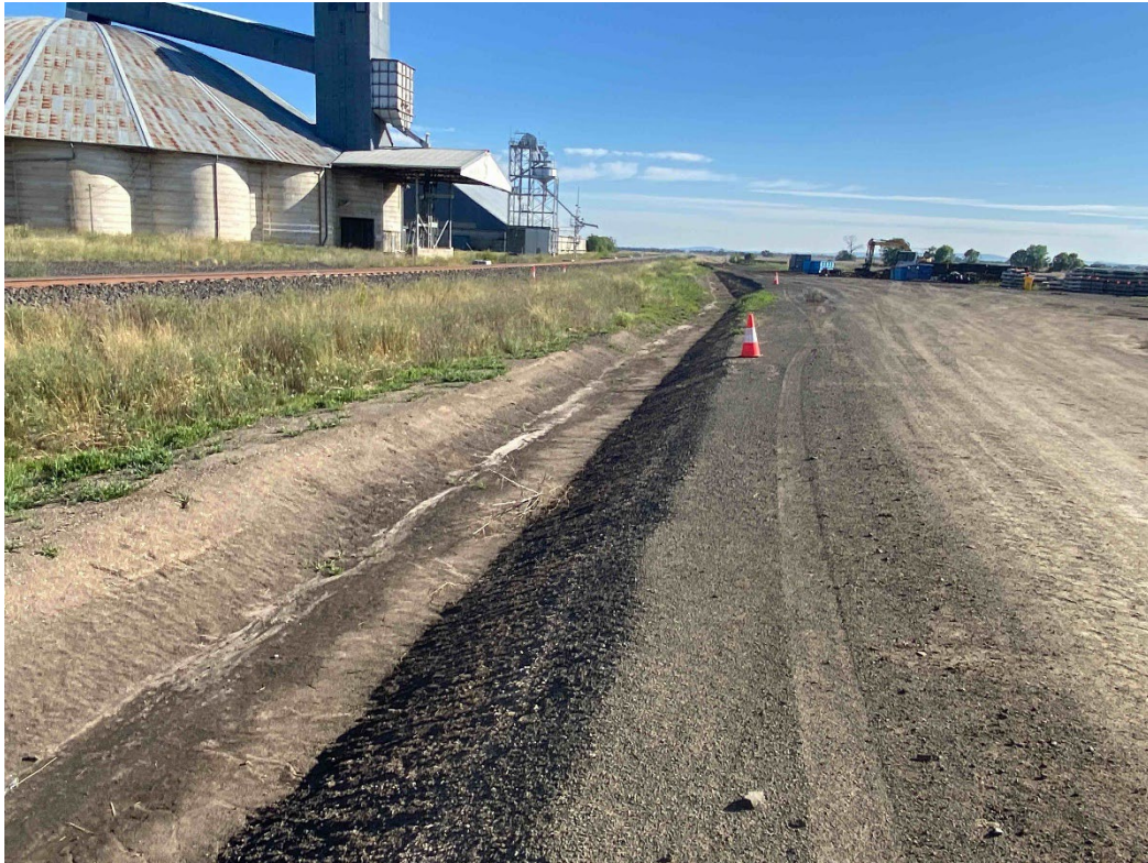
Plate 19 – Drainage channel at Milguy MAF with no scour protection
