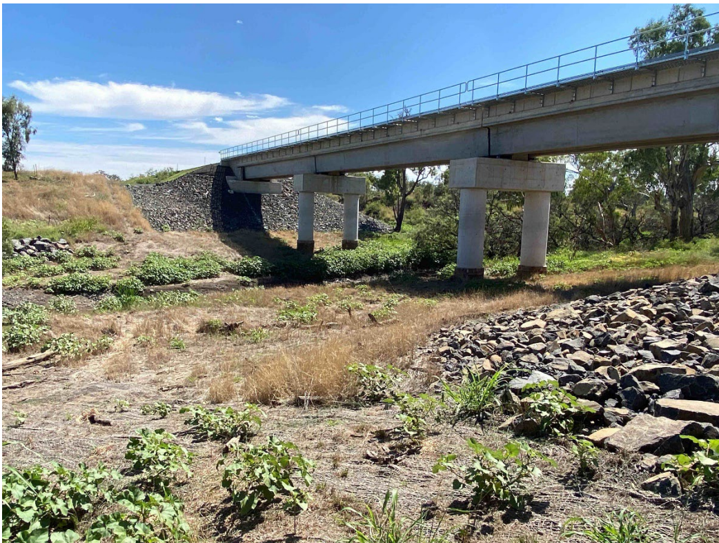
Plate 24 – Croppa Creek Bridge with jute mesh applied for slope stabilisation
