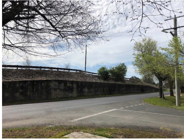
The urban interface created by the existing road bridge structure. The retaining wall directly abuts the northern kerb of Mackellar Street and causes a drainage trap point during high intensity rain events.
