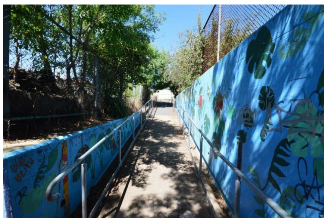
Pedestrian ramp and associated retaining wall structures when ascending from the underpass connecting Railway Place and Mackellar Street.
