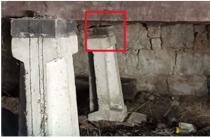
Image 3-41 – Concrete stump rotated and disconnected from bearer
