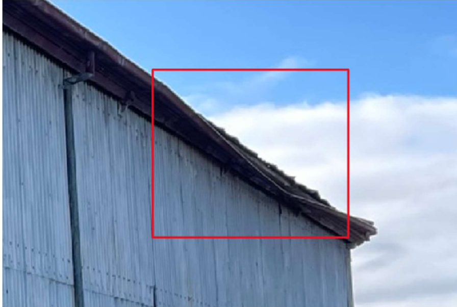
Images 3-19 – Failed gutter on Up Side
