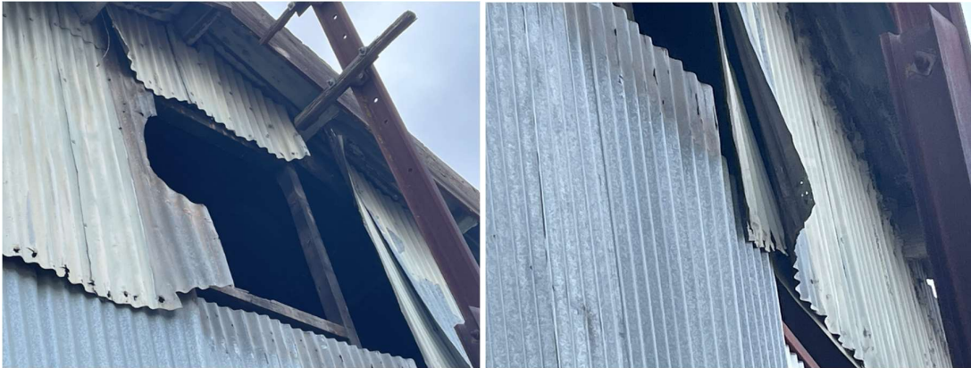
Images 3-4 & 3-5 – Failed wall sheeting on the Up End, and warped disconnected wall sheeting
