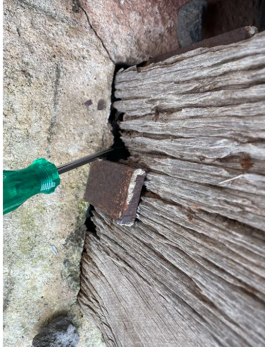
Image 3-26 – Rotten column at footing connection, Up End , Up side corner
