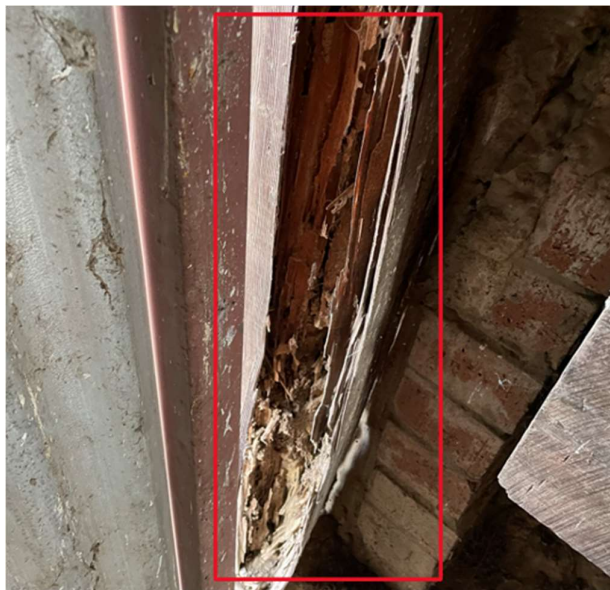
Image 3-27 – Suspected termite affected column, Up end, central
