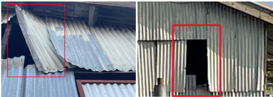
Images 3-6 & 3-7 – Precarious façade sheeting on Up End(Left image), and Down End (Right image)
