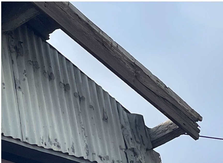
Images 3-15 – Missing roof sheeting at Up End, Up Side corner
