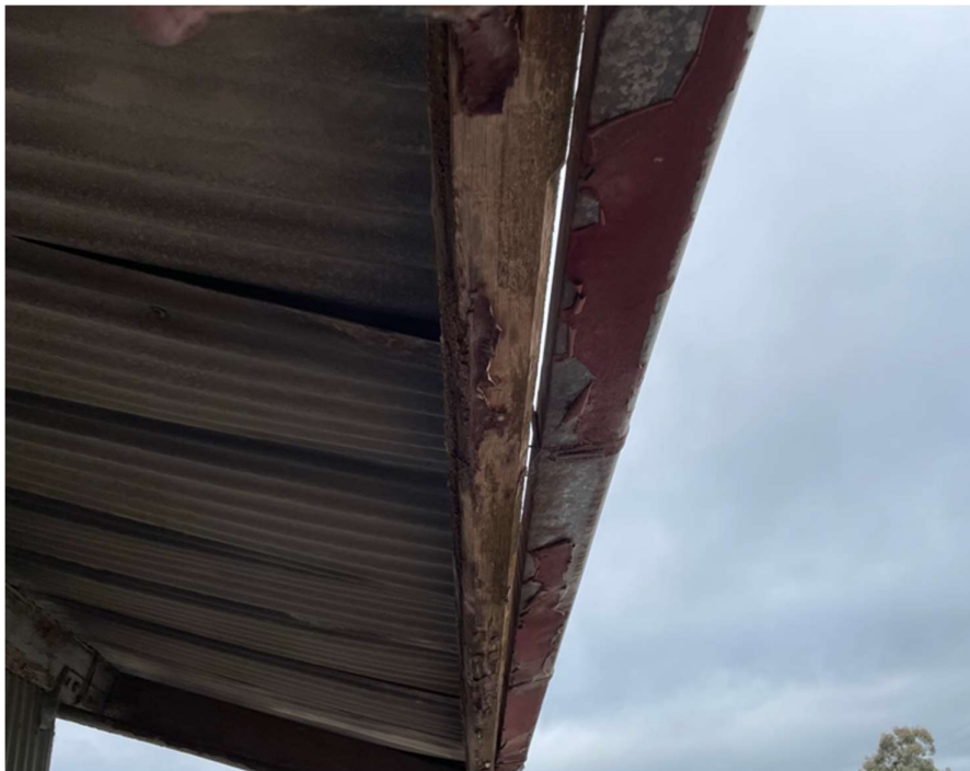
Images 3-20 – Typical condition of gutter
