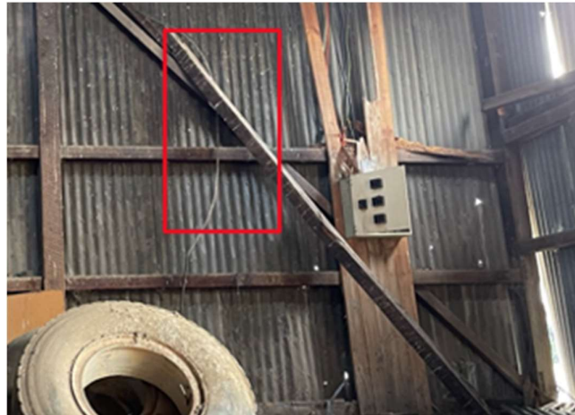
Image 3-33 – Collapsed roof bracing. Down Side, Down End
