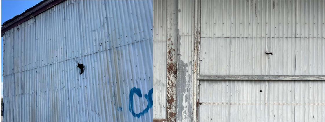
Images 3-8A & 3-8B – Typical wall cladding condition on Down Side and Up Side elevations
