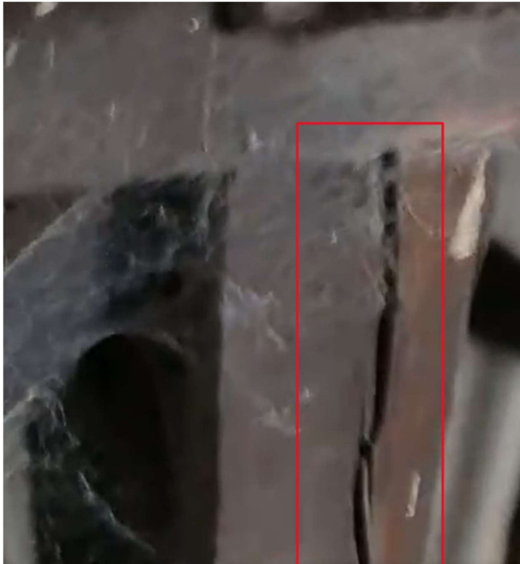
Image 3-29 – Severe split in column propagating from connection to steel roof truss Up Side
