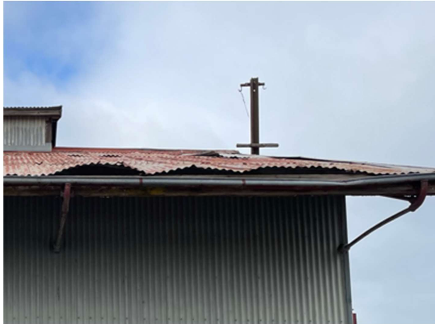
Images 3-16 – Disconnected, warped roof sheeting
