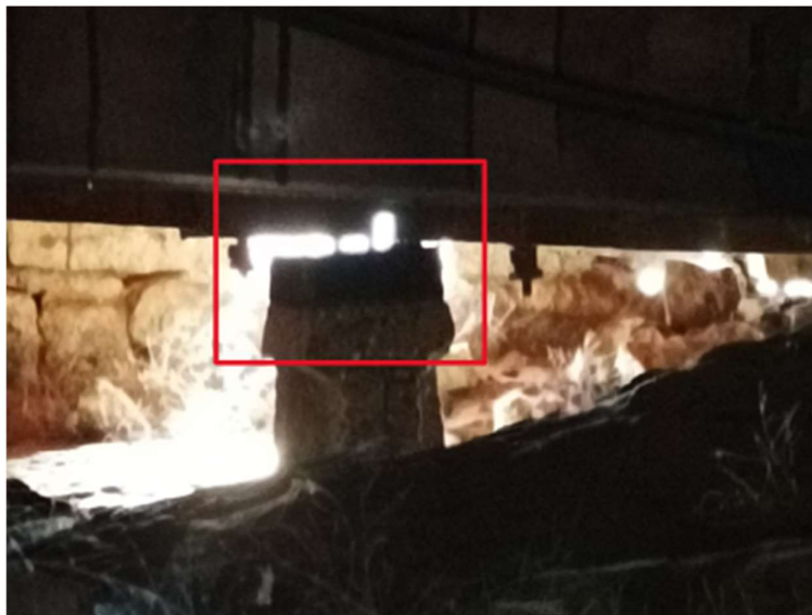
Image 3-42 – Concrete stump rotated and disconnected from bearer
