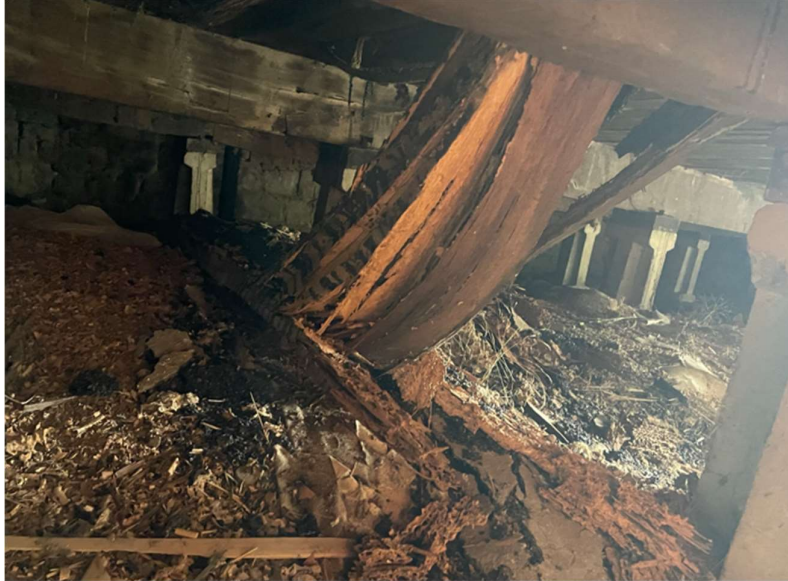
Image 3-39 – Failed timber deck poses a serious risk of injury
