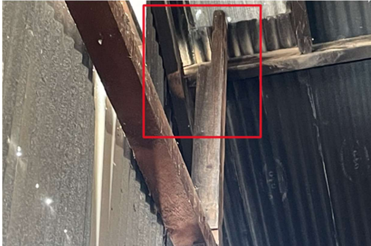
Image 3-28 – Column has disconnected from roof truss and purlin, and is leaning inwards pulling the wall beam
