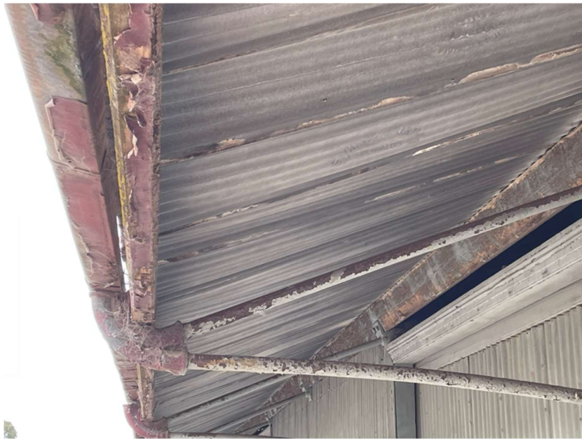
Images 3-18 – Typical condition of fascia
