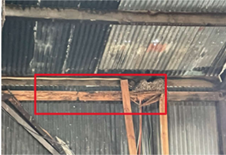
Image 3-32 – Failed timber beam at Down Side, Down End
