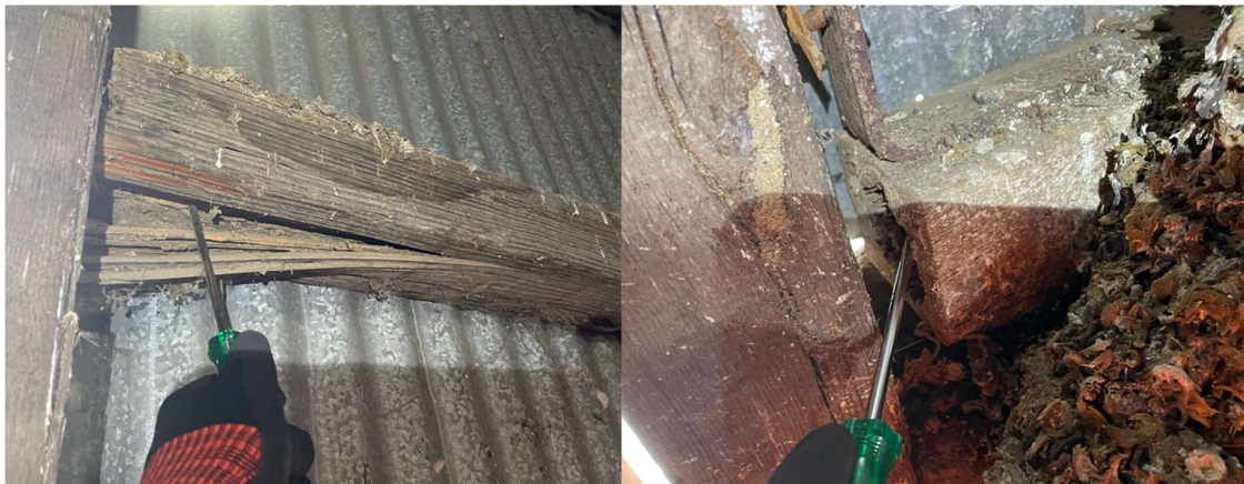
Image 3-9A&3-9B – Deteriorated timber 'girts' Up End
