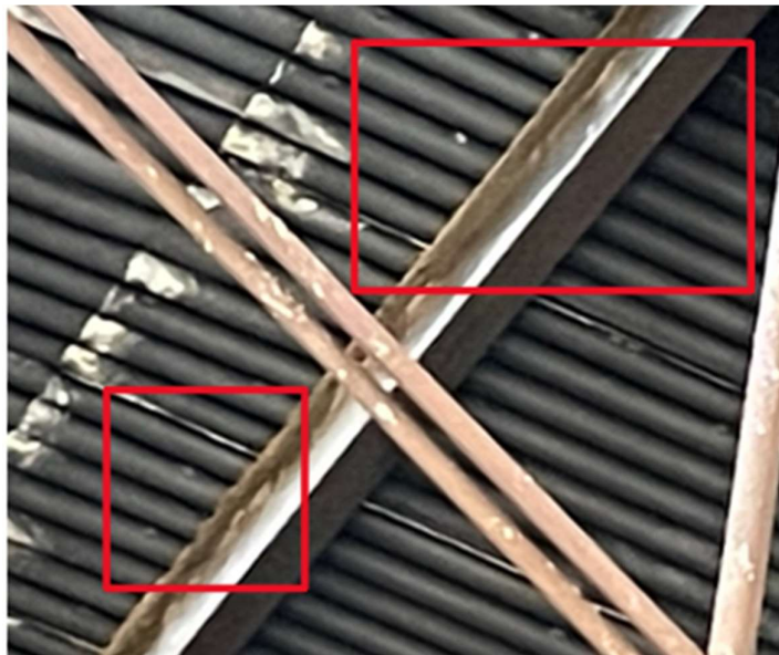
Image 3-24 – Water staining on the upper portion of purlin
