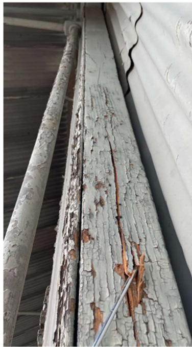
Image 3-25 – Typical condition of timber columns
