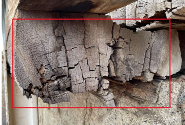
Image 3-34 – Severely split beam end, Down Side, central
