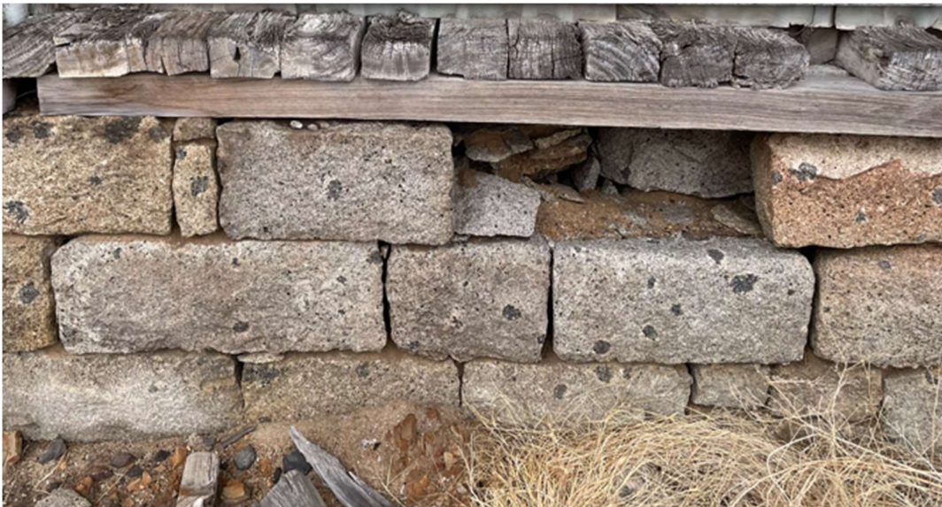
Image 3-36 – Deteriorated stone upstand, Down Side
