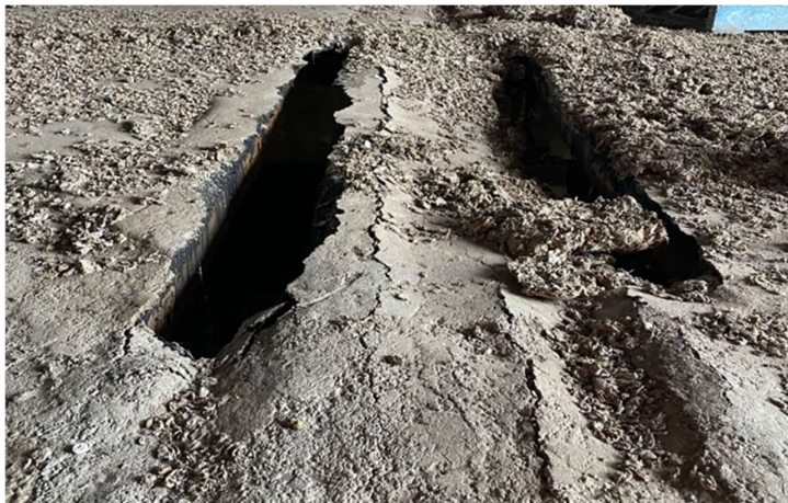
Image 3-38 – Failed timber deck poses a serious risk of injury
