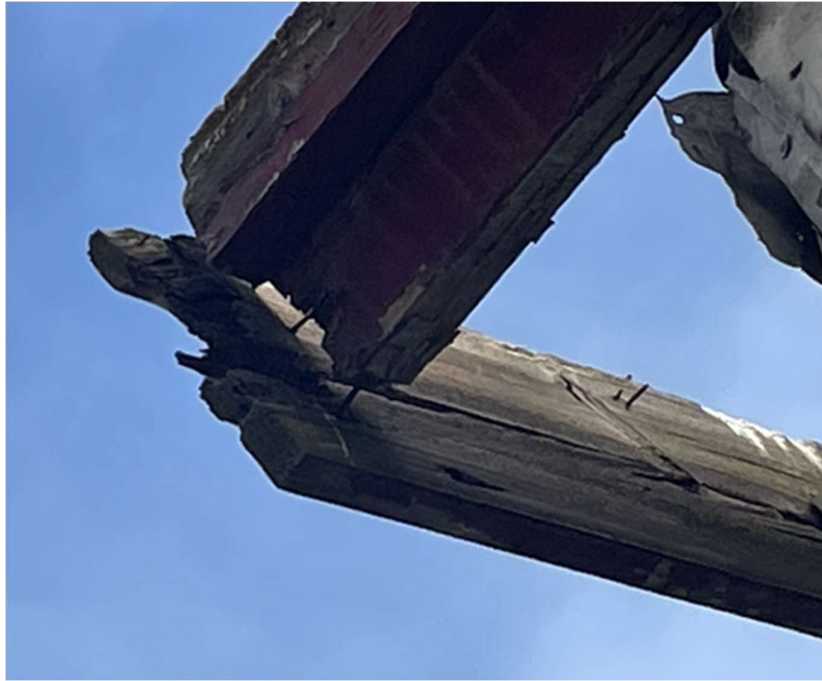
Images 3-17 – Failed fascia at Up End, Up Side corner
