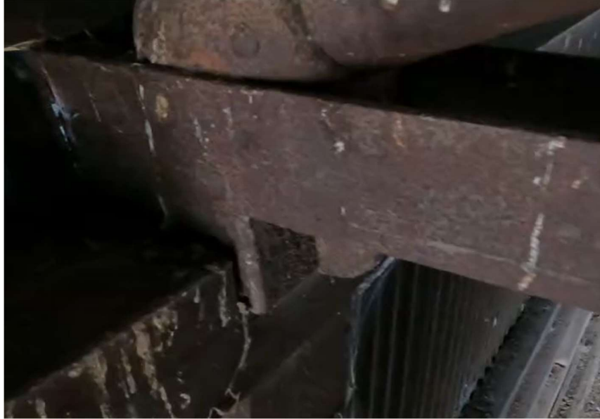
Images 3-12 – Steel roof truss connection to timber beam (image taken via Go-Pro on pole)
